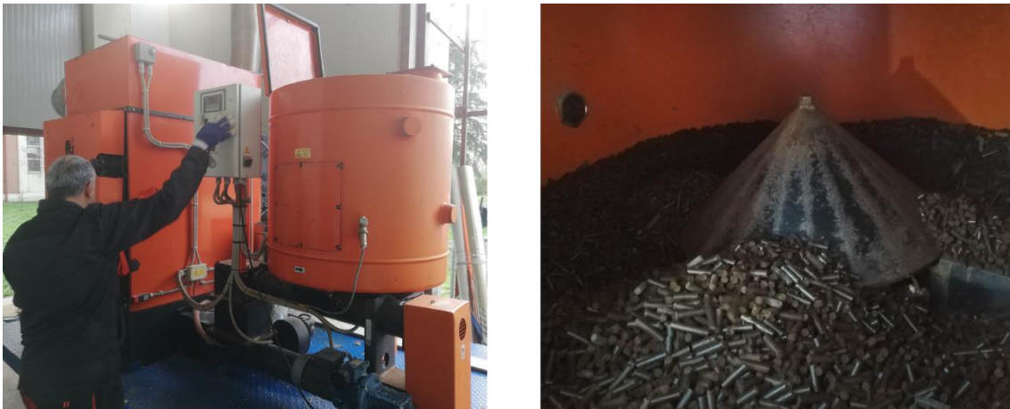
Figure 11 - on the left, the boiler used for the tests; on the right, the pellets inside the tank.
