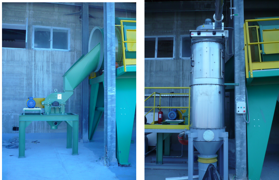
Fig.11 Hammer mill (left) and socks type aspirating filter (right).
