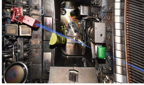
Figure 4.5: In-vessel components of the THB and the gas-puff imaging (GPI) system at the LFS in segment 13. One thermocouple used for this check is installed in the valve system which is indicated in green. Additionally, the optical head is indicated in red, the corresponding LOS distribution in blue and the GPI system in yellow. Taken from Ref. [Gri18].
