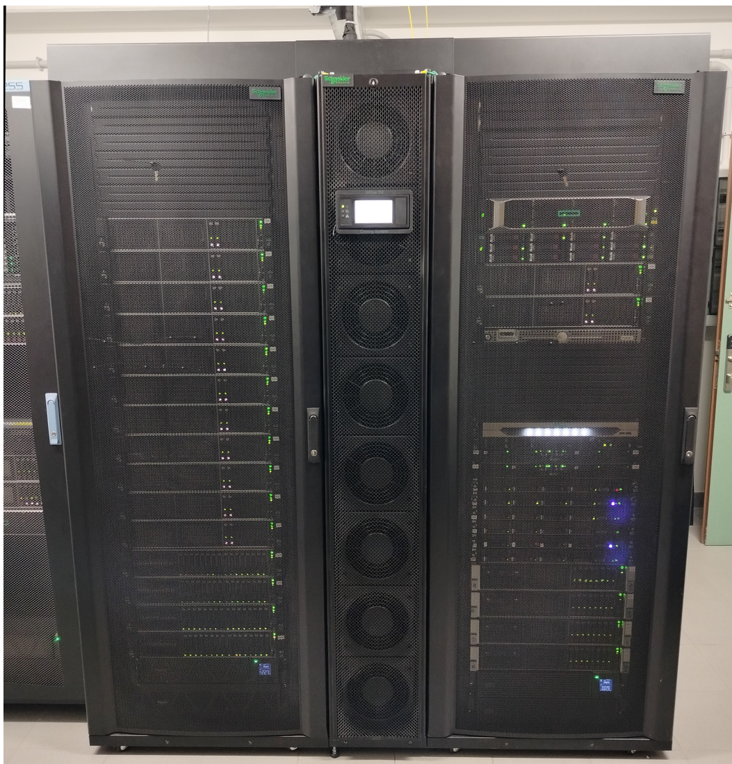
Figure 1.1: Racks with In-Row Cooling system
