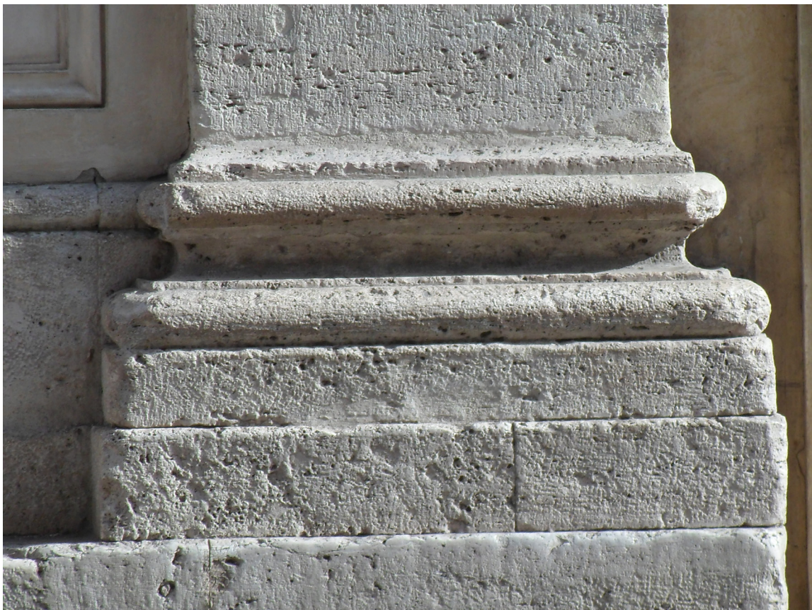
Fig. 13.1 13 The bases of S. Stanislao facade (fot. M. Hirsch) The capitals and the bases of Palazzo della Sapienza courtyard (fot. M. Hirsch)
